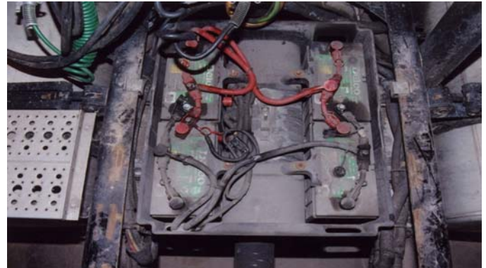
Photo 8 – Batteries Inside Frame Rails, Freightliner Century Class
